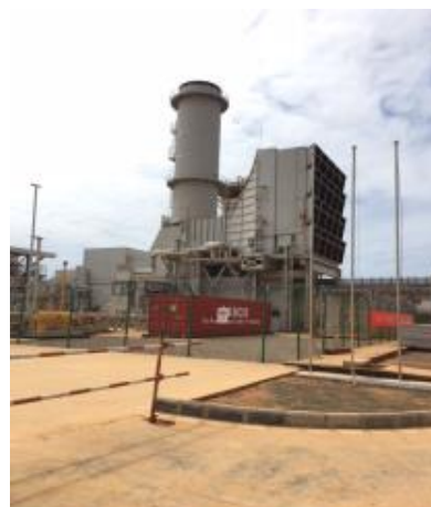
No. 4 gas turbine
