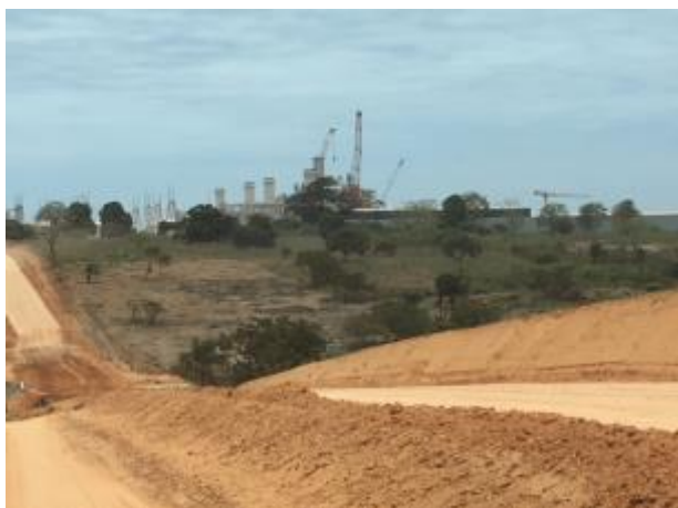
View of Soyo 1 CCGT from the access road
