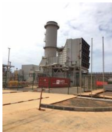
Turbina a gás No.4
